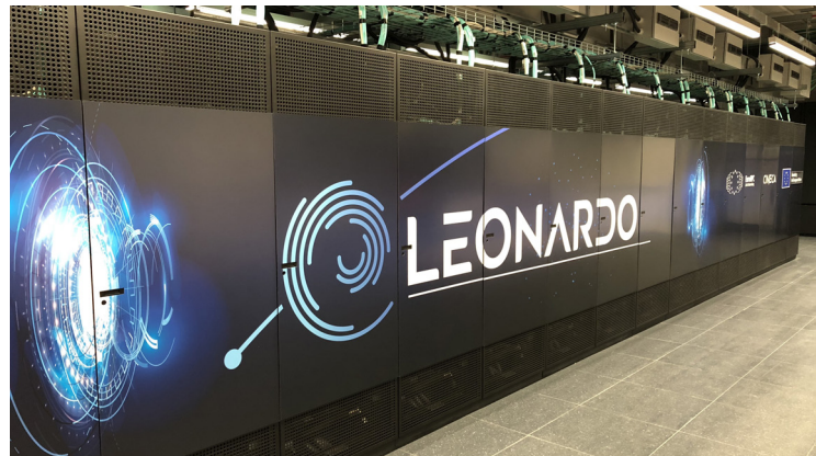
Fig. 1: Actually installed LEONARDO.
